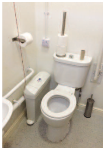
Above: Bad – the only easily visible features to the ageing eye are the toilet roll holders, brush holder, toilet paper tube and the emergency pull!
